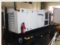
Hydraulic Power Supply (P-8)
