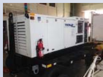
Hydraulic Power Supply (P-8)
